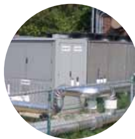
Smardt air-cooled performance at this Florida university delivered the expected 40% energy savings.
